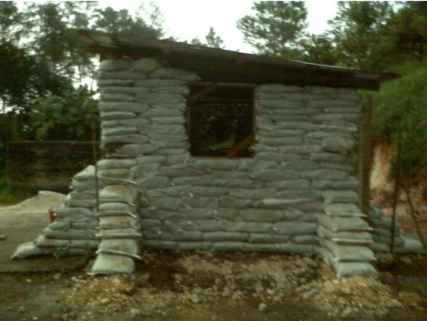
East side of house with rubble fill at base.
